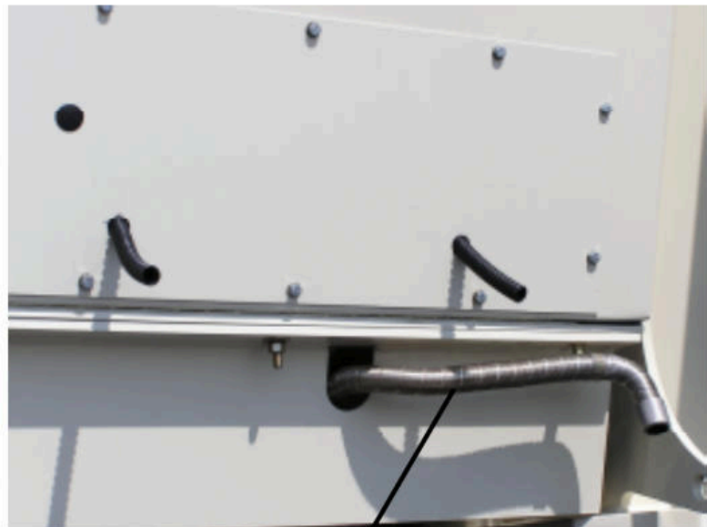
Heater Exhaust (Rear of Cab)
